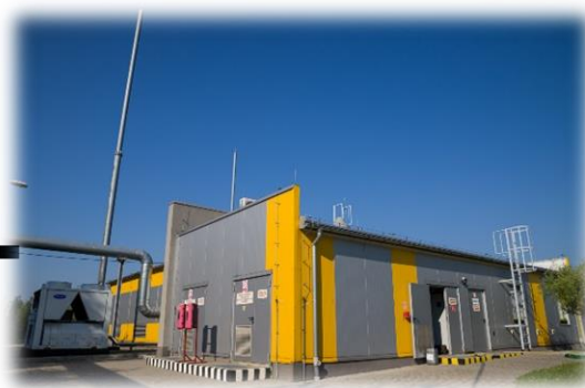
Low-concentration methane system. Drainage station
